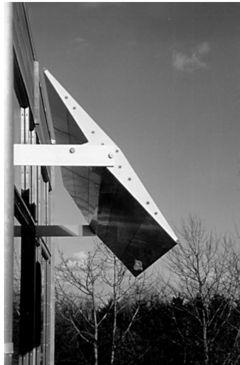
External semi-reflective light shelf in a downward-tilted position
