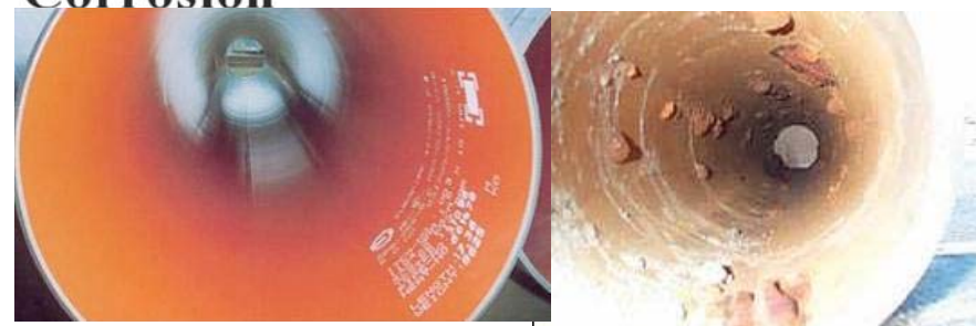
Fig. 2. Comparisons of the newly and corrosion pipes
